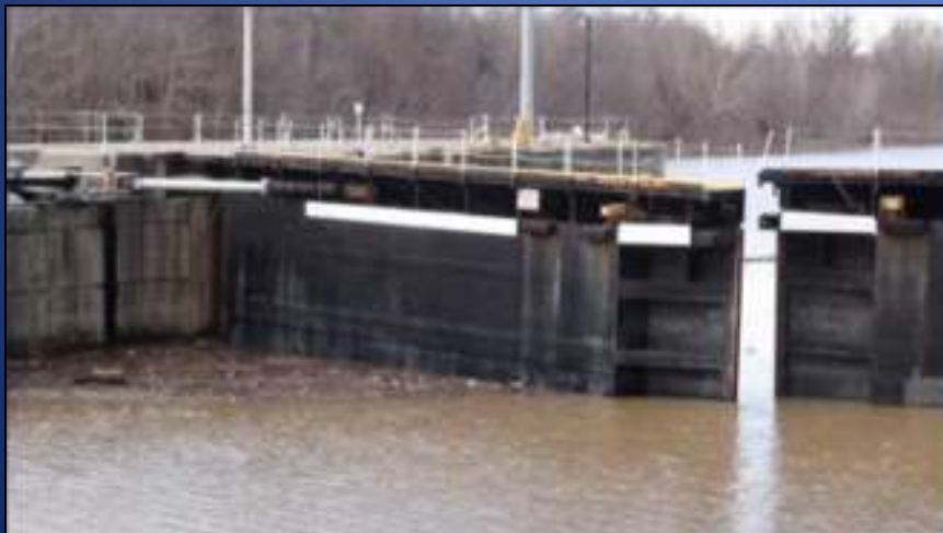
Greenup main chamber downstream gate drops 1.2 feet when anchorage fails.
