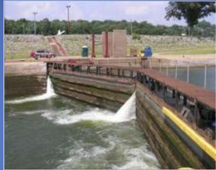
Leaking miter gates, Lock & Dam 52, Ohio R.
