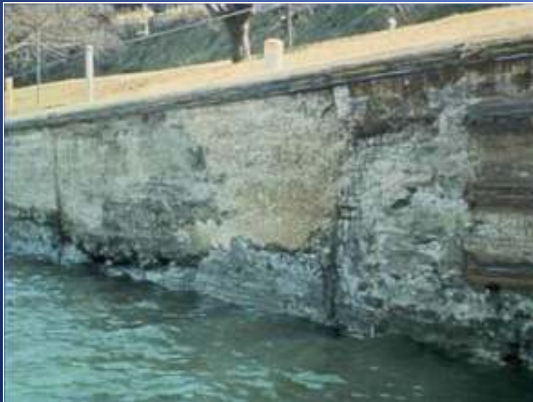
Crumbling lock wall, Lower Mon 3, opened in 1907
