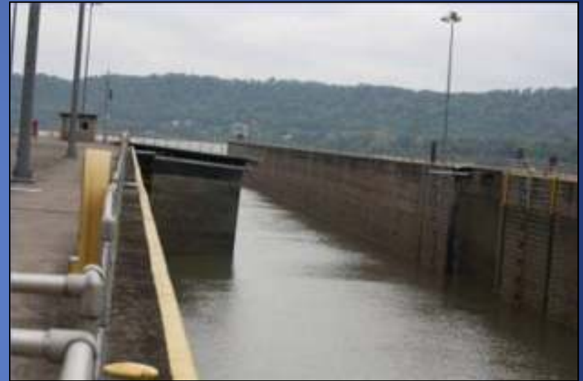
Markland main chamber downstream gate leaf has collapsed into river.
