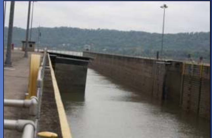
Markland main chamber downstream gate leaf has collapsed into river.
