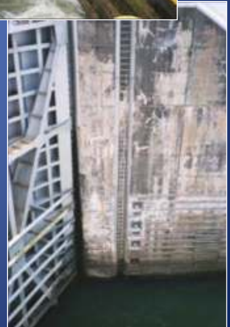
Concrete deterioration at Chickamauga could result in lock failure
