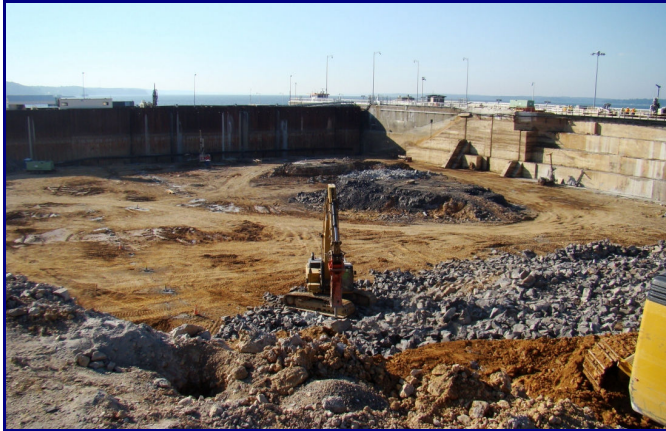
Excavation at the Kentucky Lock Addition Construction Site where as of November approximately 50 feet of material had been removed
