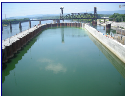
Completed Cofferdam at the Chickamauga Lock Project Site that will be pumped dry in the coming weeks. At that time construction is scheduled to be suspended for what could be as much as a decade without a resolution of the insolvency of the IWTF.
